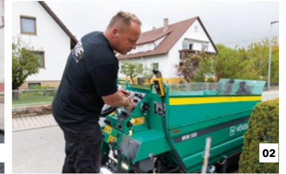
01 MINI pavers are outstandingly suitable for paving asphalt between tracks or in milled tracks.
